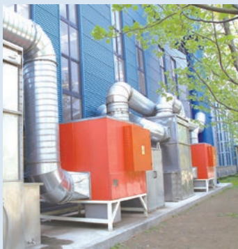
Mobile welding smoke room
